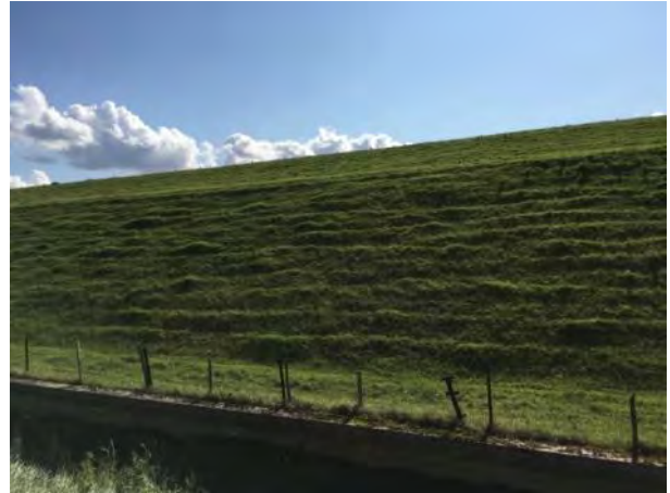
Sheep trails on steep reservoir embankment.
